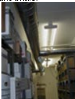
The new system keeps the Archives Room at 68 degrees and 45% relative humidity year round.
